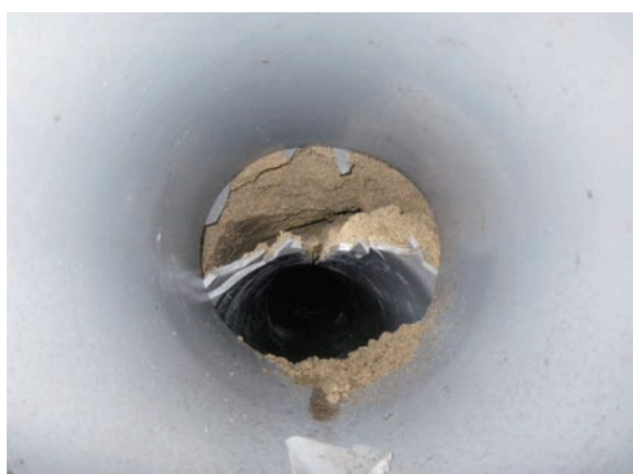
The chloroethene pipe broken by the earthquake
