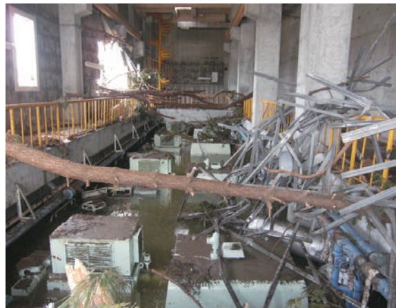
Inside of the blower room
