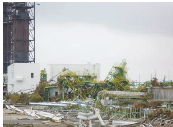
The damaged primary sedimentation tank
