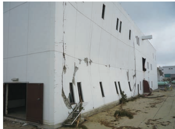
The 3 rd pumping building with the wall curved by the tsunami
