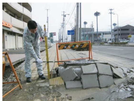
The floating manhole by liquefaction
