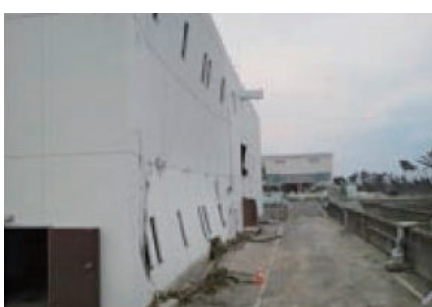
津波の衝撃により壁面が湾曲した第三ポンプ場 Dented wall of the third pumping station building due to the impact of the tsunami
